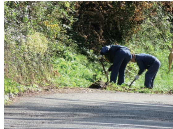
Cleaning up mud from side grooves of a prefectural road near Toda Pigment Corp.
