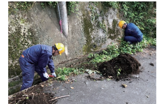
Cleaning up mud from side grooves of a prefectural road near Toda Pigment Corp.
