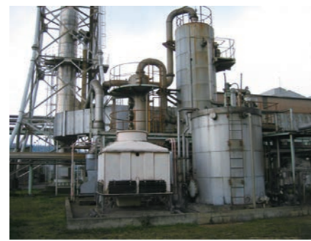
Sodium carbonate manufacturing plant
