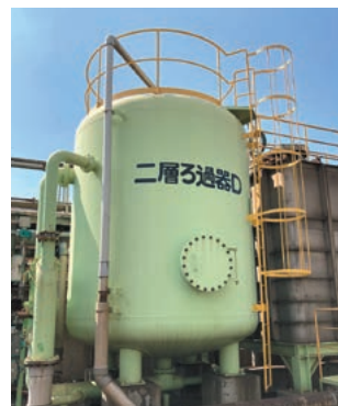
Filtration system (at the Onoda Plant)
