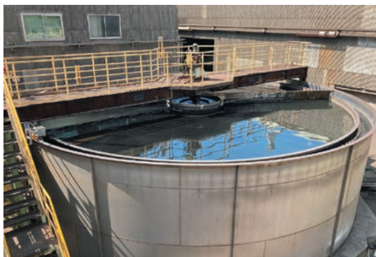
Wastewater treatment facility (at the Onoda Plant)
