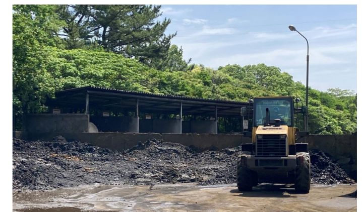
Recycling of sludge (at the Onoda Plant)
