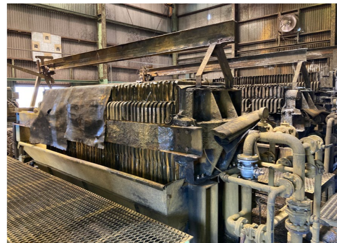
Wastewater treatment filter press (at the Onoda Plant)
