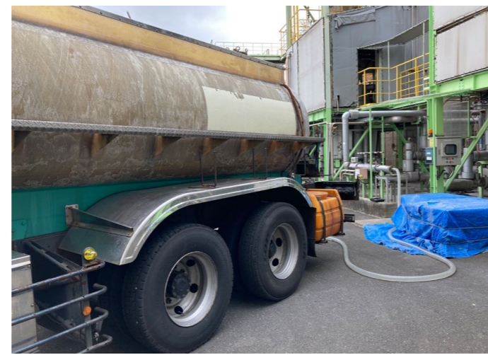
Facility for loading barium-containing effluent (at the Onoda Plant)
